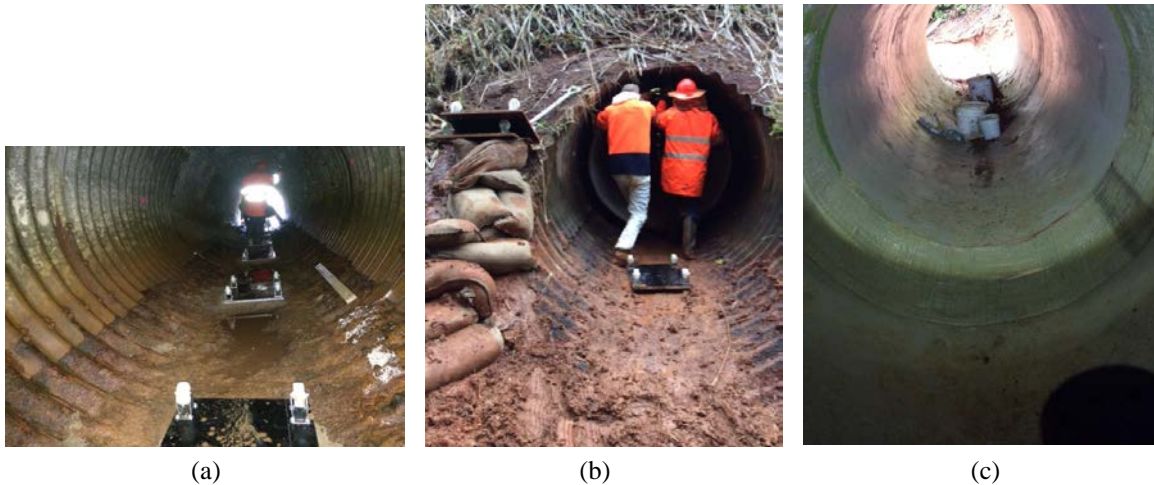
Fig. 6. (a) Caster trolleys inside the culvert allowed pushing lightweight StifPipe® segments by hand into the culvert (b); (c) joining of segments with wet layup
