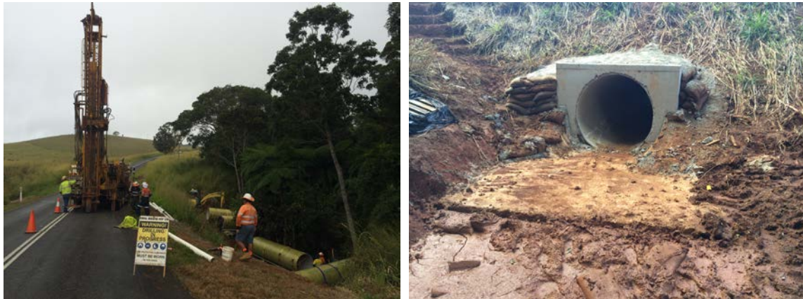
Fig. 7. Coring of the roadway for placement of grout and the finished headwall
