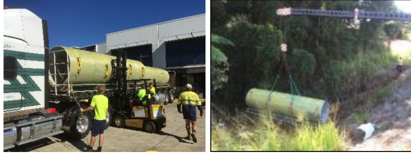
Fig. 5. Transportation of the pipes to the site and placement by the culvert
