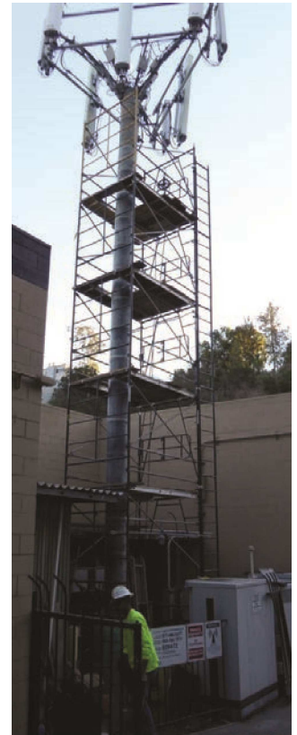
Fig. 7: Retrofitted pole prior to the application of paint and removal of the scaffolding
