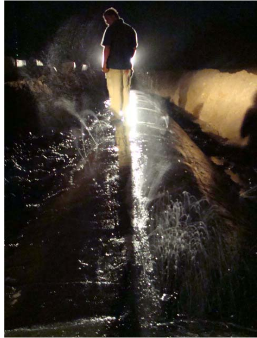
Figure 2: Leaking after conventional crack sealing
