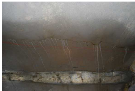
Figure 3: Water seeping into pipeline
