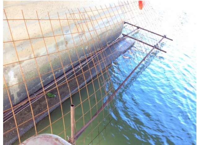
Figure 9 - Steel cage around each pier to protect the diving crew from crocodiles and bull sharks
