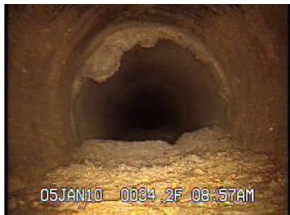
Figure 15. Heavily debris-laden pipe ID.
