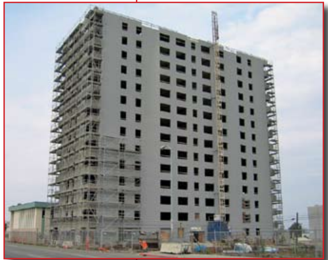
Figure 1: Damaged McKinley Tower sat vacant for more than two decades.
