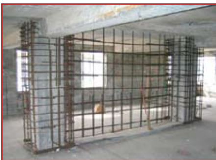
Figure 2: Original retrofit scheme required new shear walls and enlargement of existing columns.
